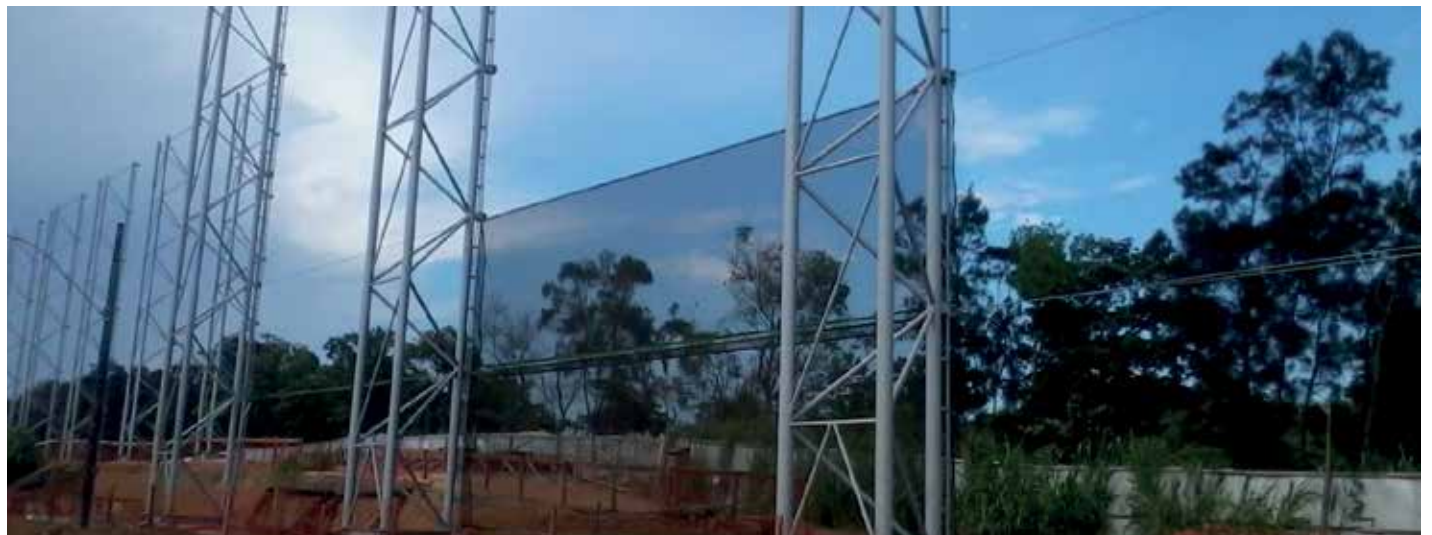
Installation of wind fences in the pellet and pellet feed stockpile yards - Ubu
